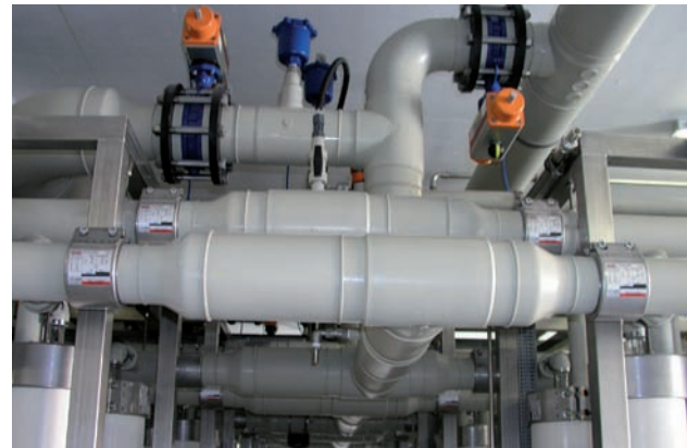
Water treatment application; connections between the racks
