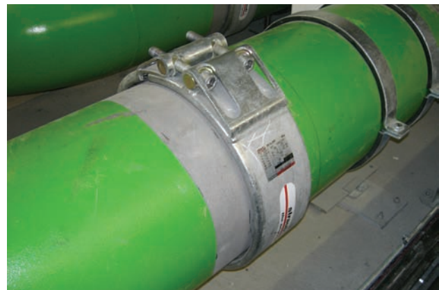
Cooling pipeline of an engine test facility with a working pressure of 6 bar and a temperature up to 60°C
