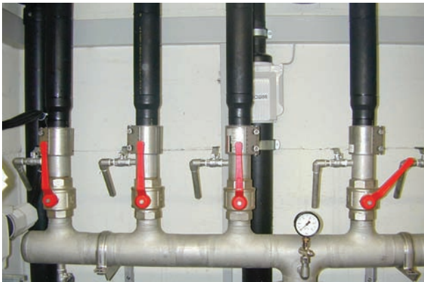
Connection of PE and stainless steel pipes, which have been installed in a well room
